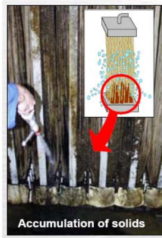
Membrane fouling at bottom
