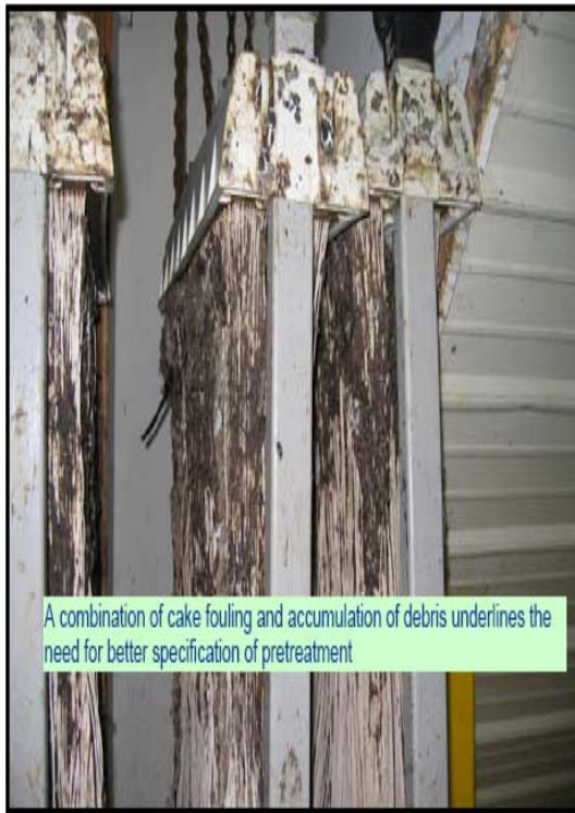
Membrane fouling at top
